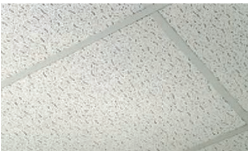
Conventional ceiling tile.
